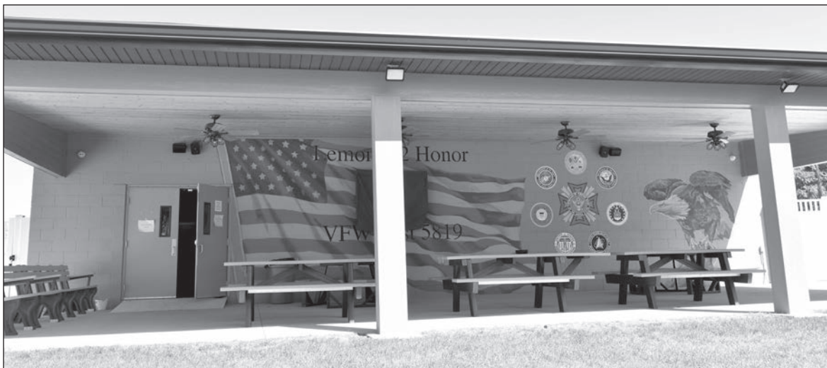
VFW Post 5819 completed work on its patio by adding a roof with lighted fans, as well as a television, so that it can be enjoyed by its members during inclement weather.
